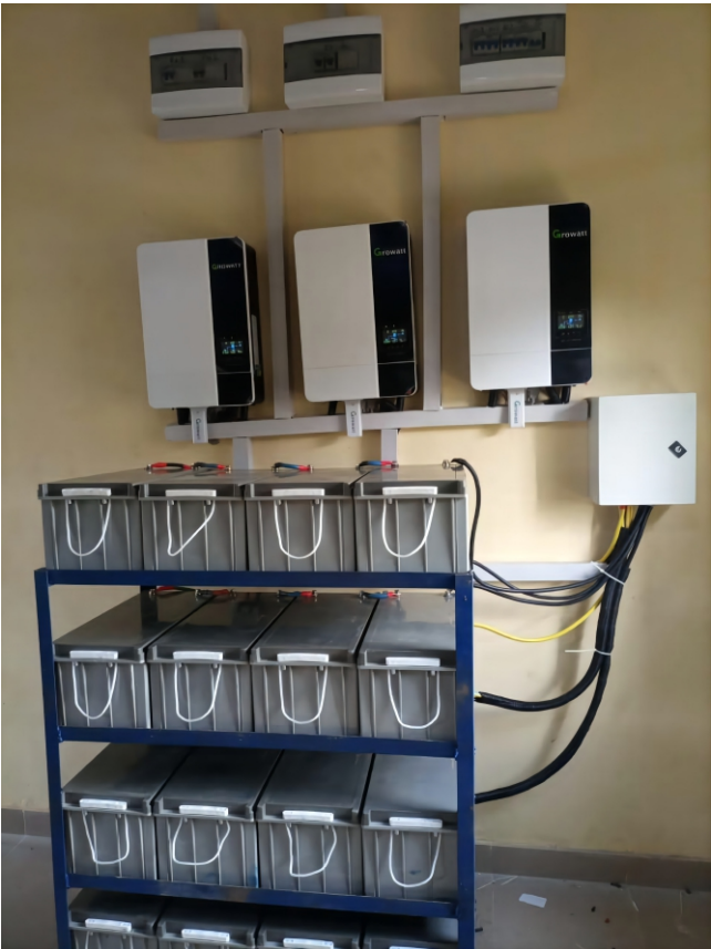
▼ 15kW three phase system ▼ Nigeria ▼ SPF 5000ES
