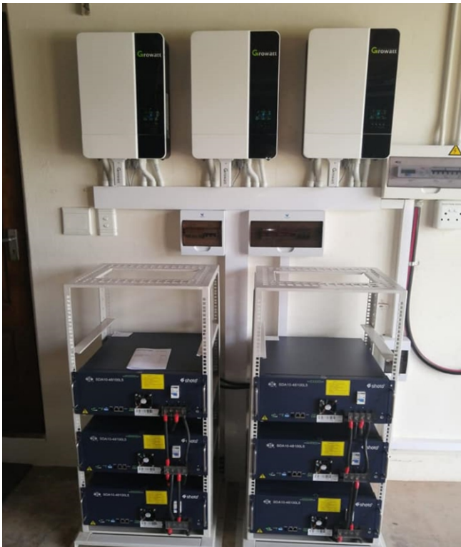
▼ 15KW Three phase system ▼ South Africa ▼ SPF 5000ES
